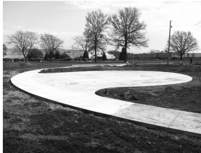
The foundation for the shelter. L.L. Geans will provide a 24' square open-air shelter with a metal roof. The park staff will place picnic tables under the shelter.
