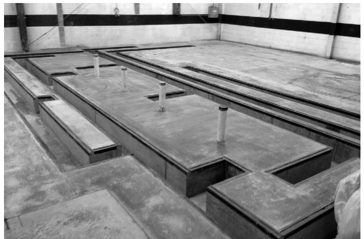
The finished project—the trench drain is ready for the installation of two aluminum die casting machines.
